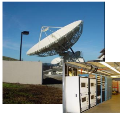
6 Ground Earth Stations
