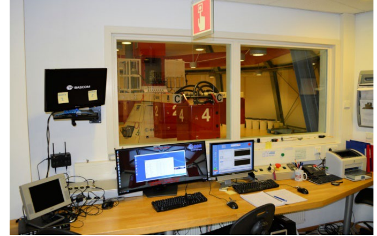
LDC control room
