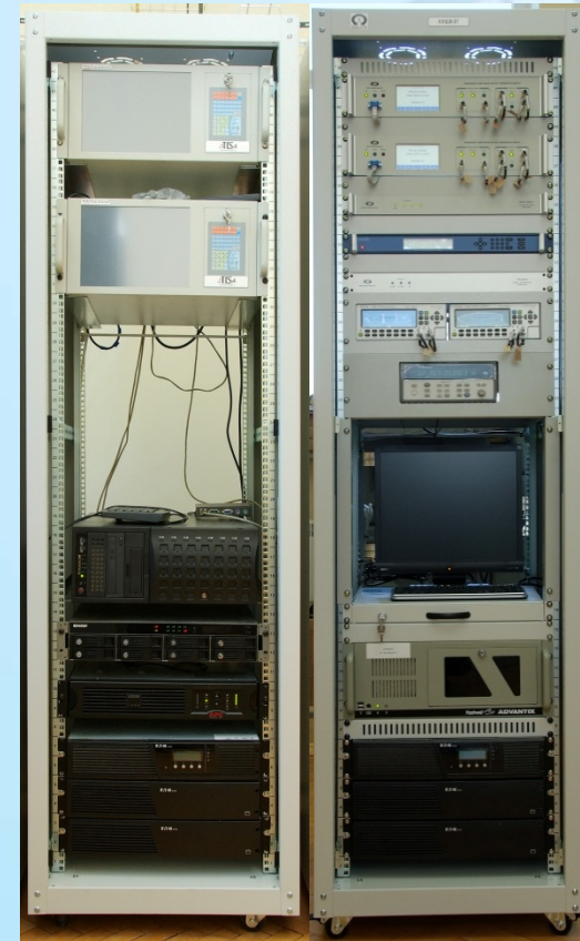
Ground Control Segment Equipment
