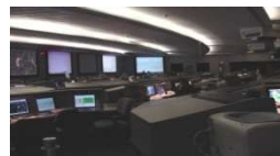
2 Operational Control Centers
