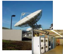
6 Ground Earth Stations
