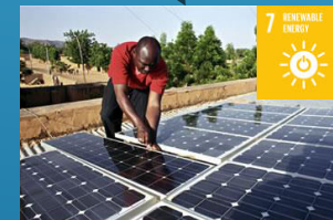
Monitor Villages electrification with Solar Panel
