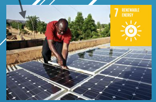
Monitor Villages electrification with Solar Panel
