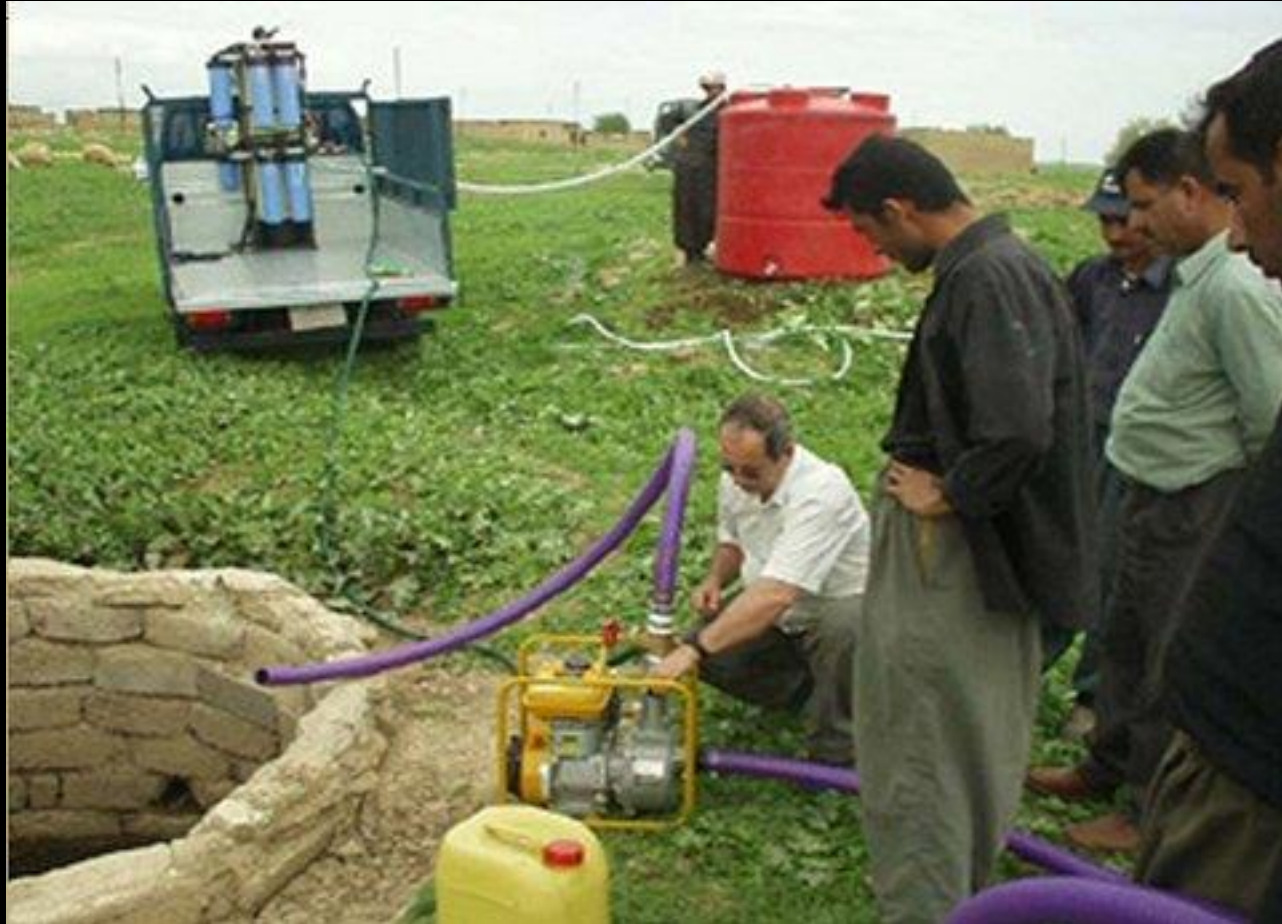
Volunteers help install and test a water purification system in Kendala, Iraq.
