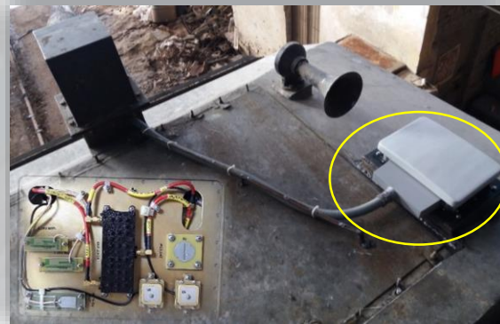
Installed Terminal – Top View
