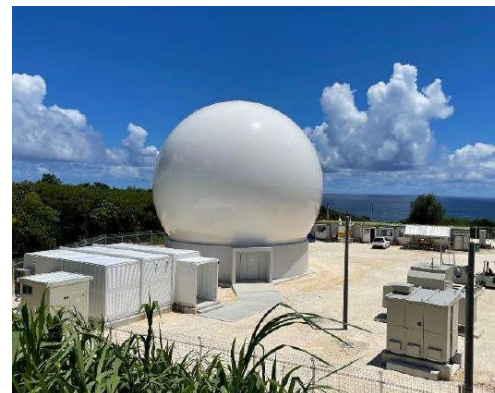
The new TT&C station at Miyakojima-island
