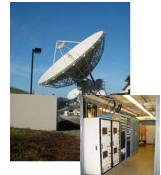
4 Ground Earth Stations
