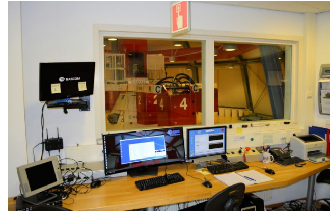
LDC control room
