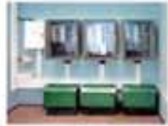
Antenna control system
