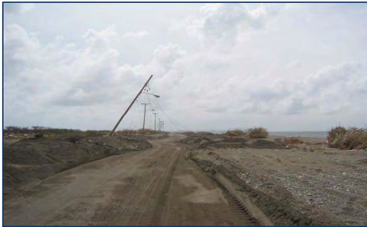
Damage to the Palisadoes Peninsula after Hurricane Ivan in 2004 (Source: wunderground)
