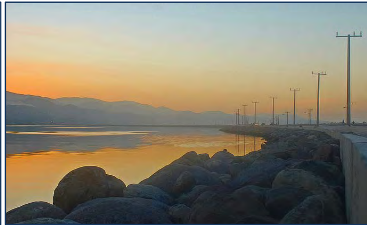
Construction of rock revetment walls after road improvement and shoreline protection work on the Kingston Harbour side of the Palisadoes Peninsula.
