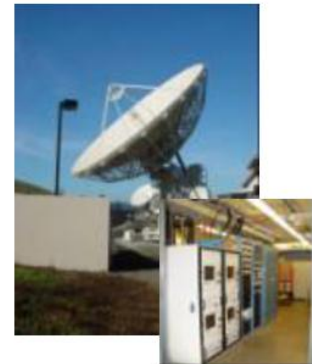
6 Ground Earth Stations
