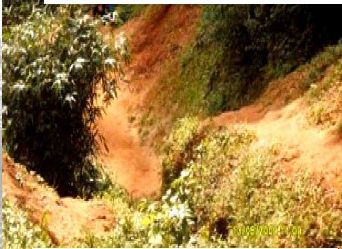
EROSION SITE IN IMO STATE
