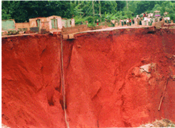
EROSION SITE IN ANAMBRA STATE
