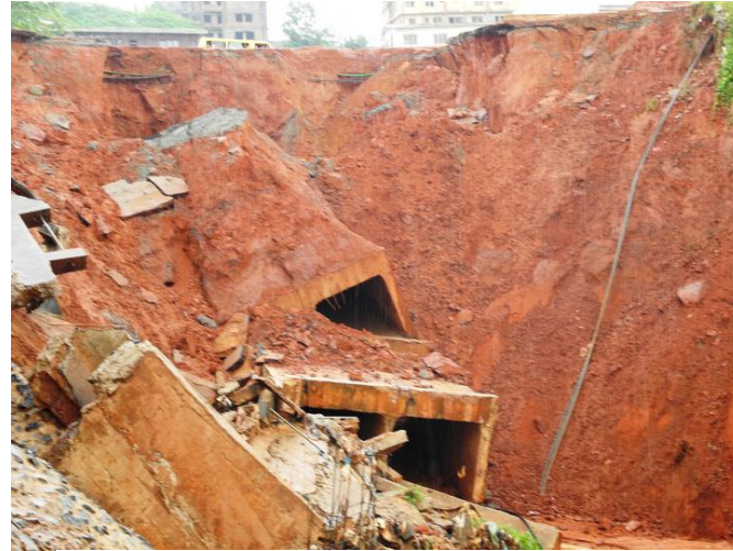
EROSION SITE IN ABIA STATE
