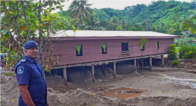
A police officer looks at the damage caused by the landslide. Photo: Department of information
