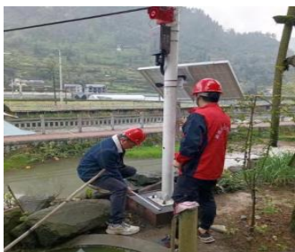
Workers installed BeiDou monitoring equipment at risky sites of geological disasters
