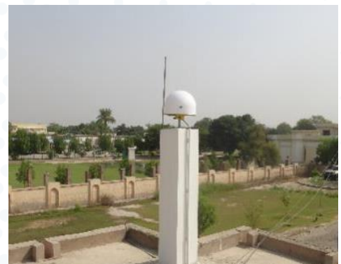
GNSS Signal Monitoring Station
