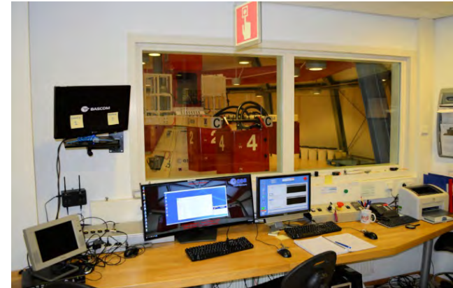
LDC control room
